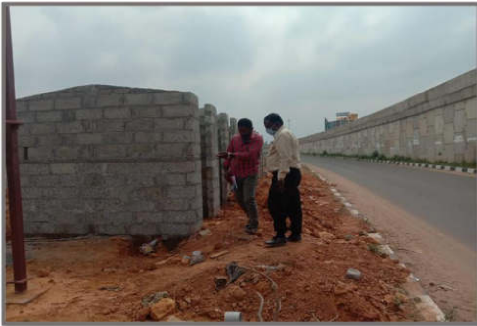
Separate rest rooms for women labourers being constructed for their health and safety.
