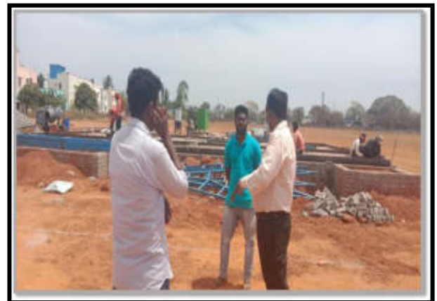
Construction Site visit by Superintending Engineer (PMU), Executive Engineer (Trichy) and Social Development Specialist (Gender)- Vallam
